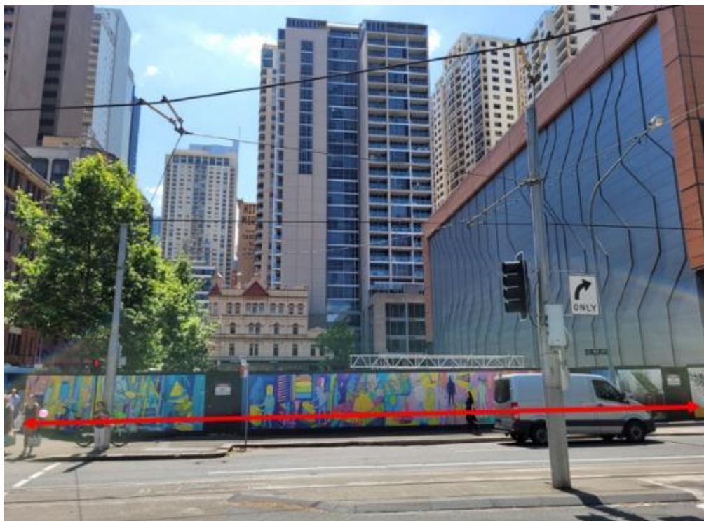
Figure 2: Site viewed from Hay Street, with the neighbouring Belmore Park Zone Substation to the right
